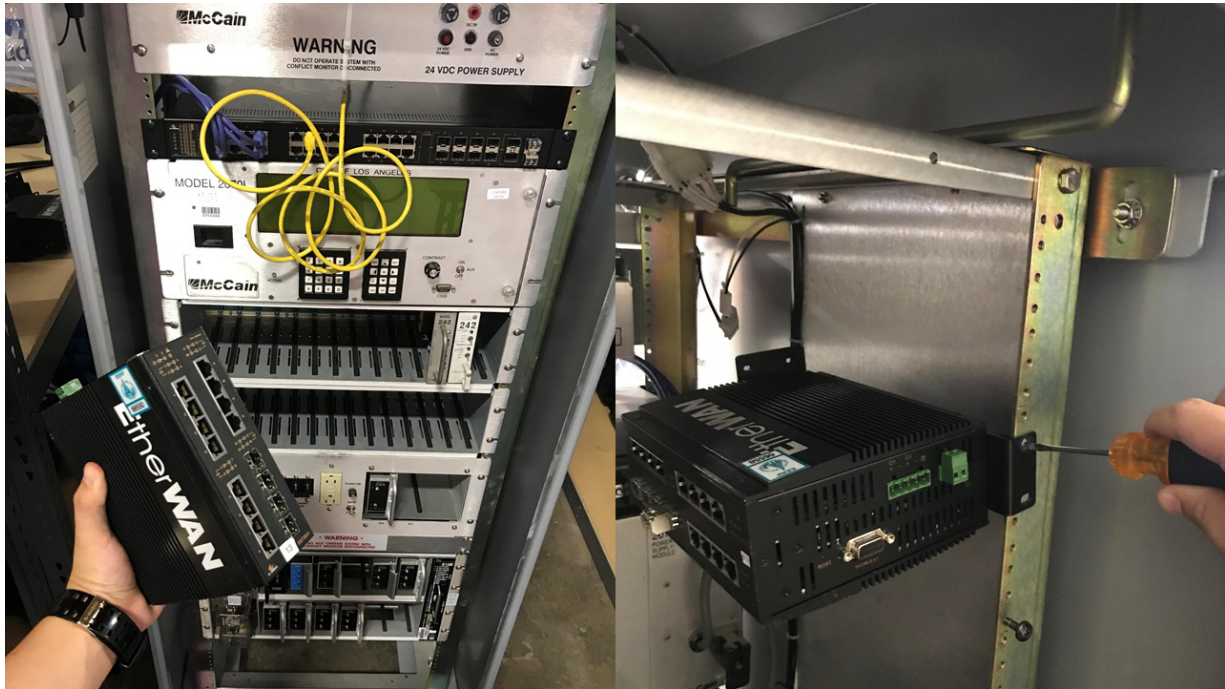
Most cabinets do not utilize the empty spaces in the back.
